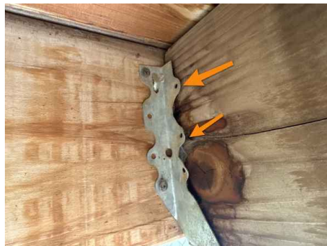
No screws in hanger
