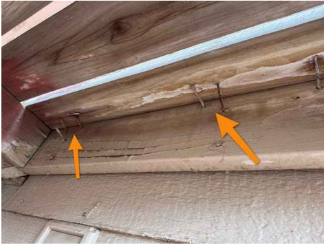
Nails backing out
